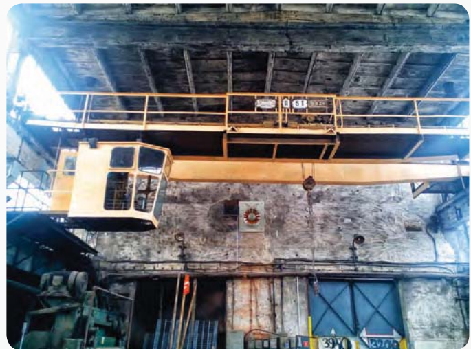
Fot. 2. Suwnica I S Photo 2. Gentry crane I S
